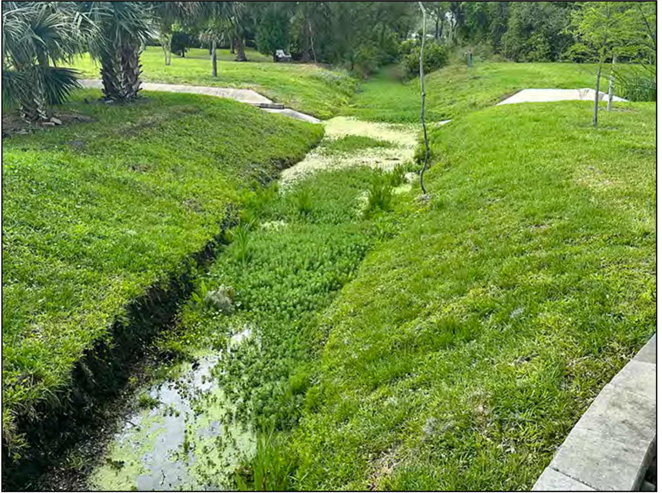
Figure No. 3 - Current ditch condition exhibiting excess aquatic vegetation, Pond #8 is to the Right and Proposed Pond #16 is to the Left in the photo.
