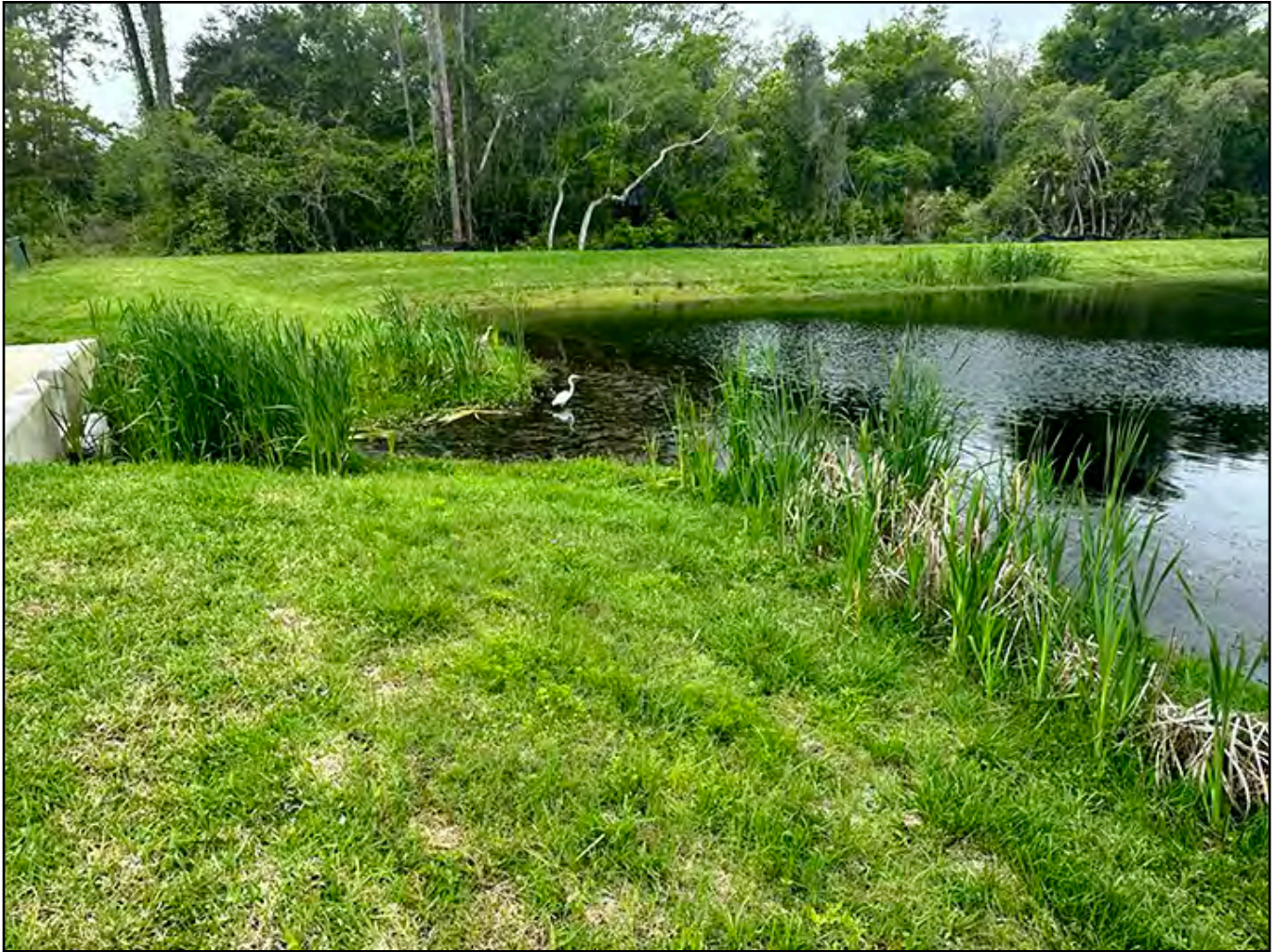
Figure No. 6 - Proposed Pond #16 conditions showing control structure blocked with vegetation.
